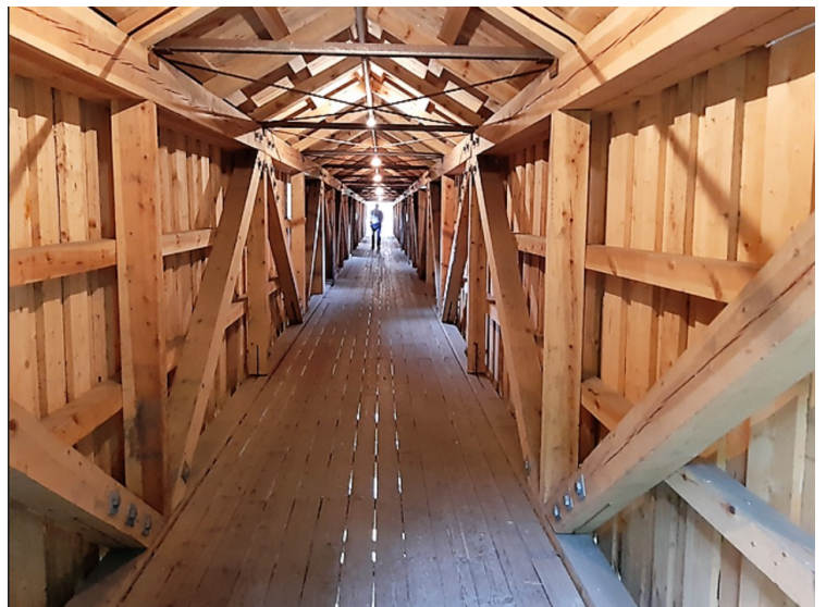
I'm on my way through the walkway to the blast furnace house.
