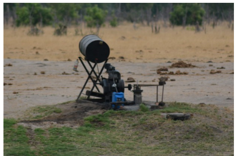
Closeup of the pump.
