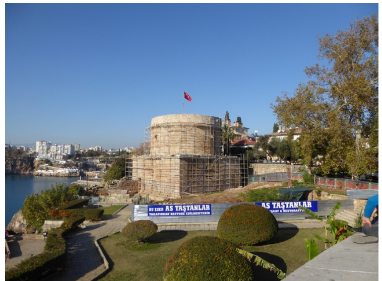
Hidirlik's tower again. There is scaffolding around the tower, so there are restoration work going on.
