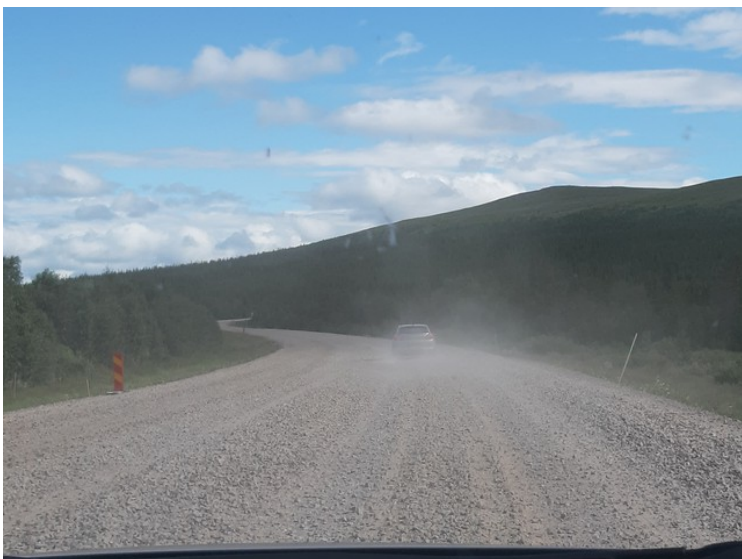
Road work was underway in many places along the E45, and then we had to drive on gravel roads like this.
