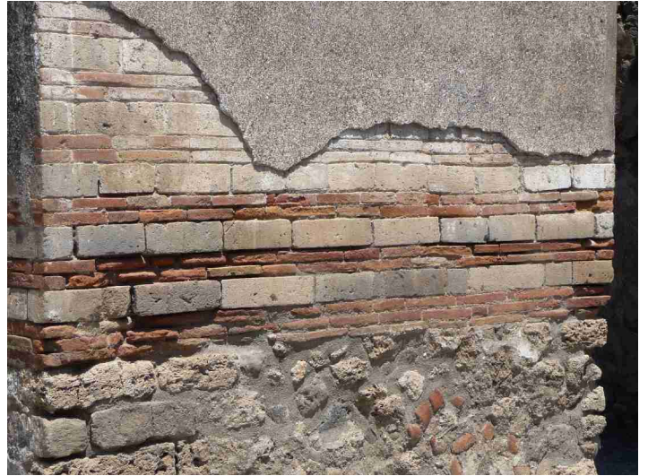
Here we can see how they laid the bricks. There was finishing mortar on top in addition.
