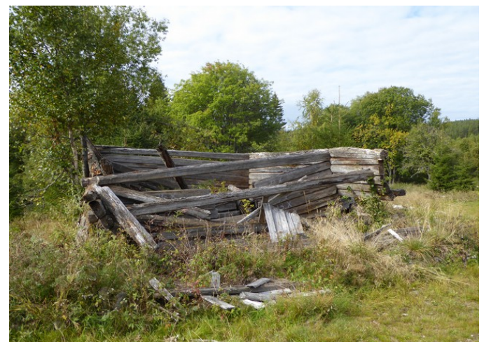
Some of the buildings are falling into disrepair.
