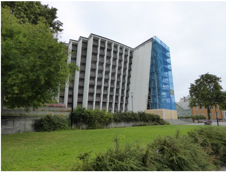
We drove up to Kirkelandet church . It was built in 1964. Maintenance was underway.
