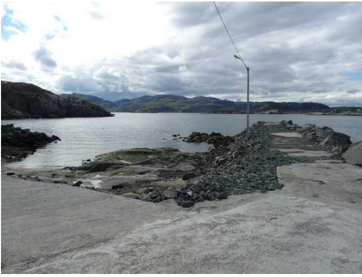
The pier has not been maintained lately.
