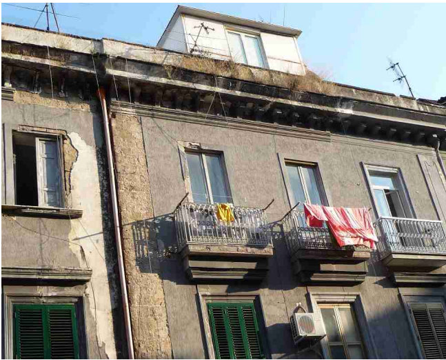
The plastering is flaking off and there is growing weeds in the rain gutters.
