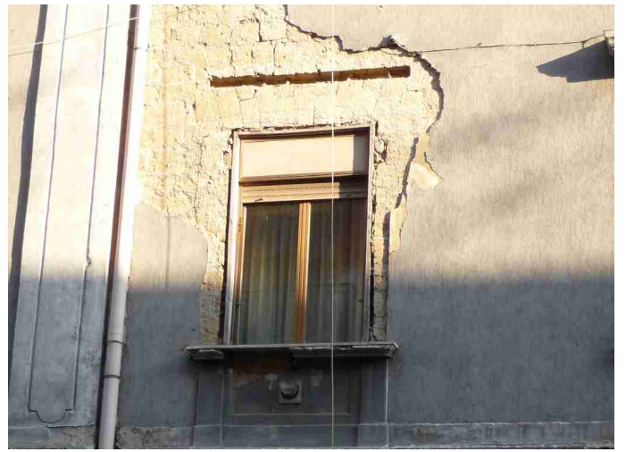
The facades were not very maintained
