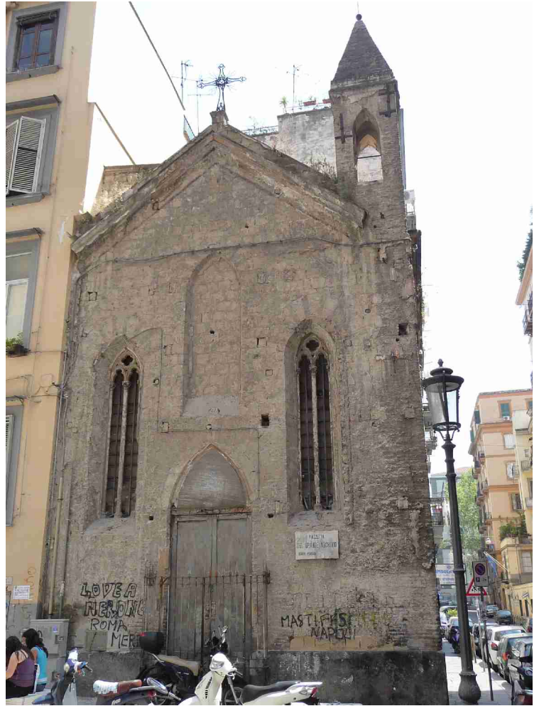
The church Santa Donna Regina Vecchia is in bad shape.
