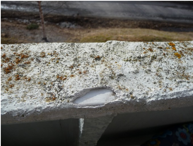
This is the railing. I removed a bit of texture paint to show the thickness. Everything is mossy.
