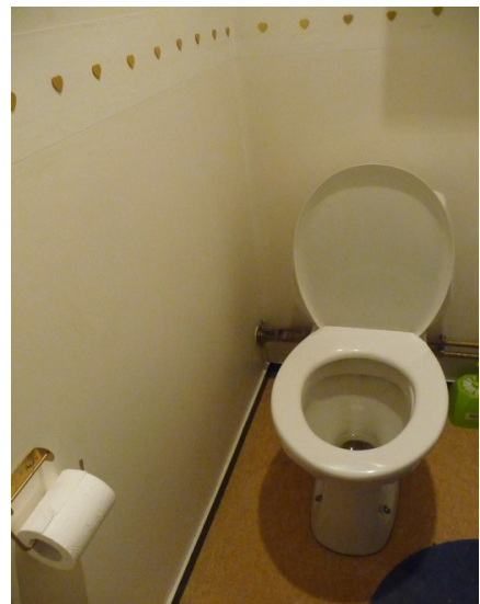
The toilet bowl was cracked.
