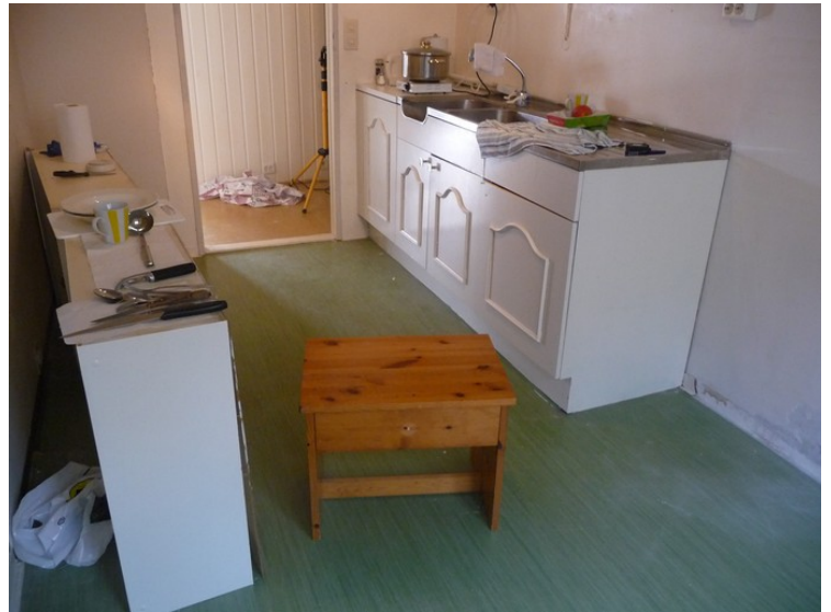
Here we are in the process of removing the cabinets. The plates on the bench was used as chopping board for many years.
