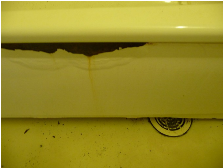
The bath tub is flaking and there is shit down the drain.
