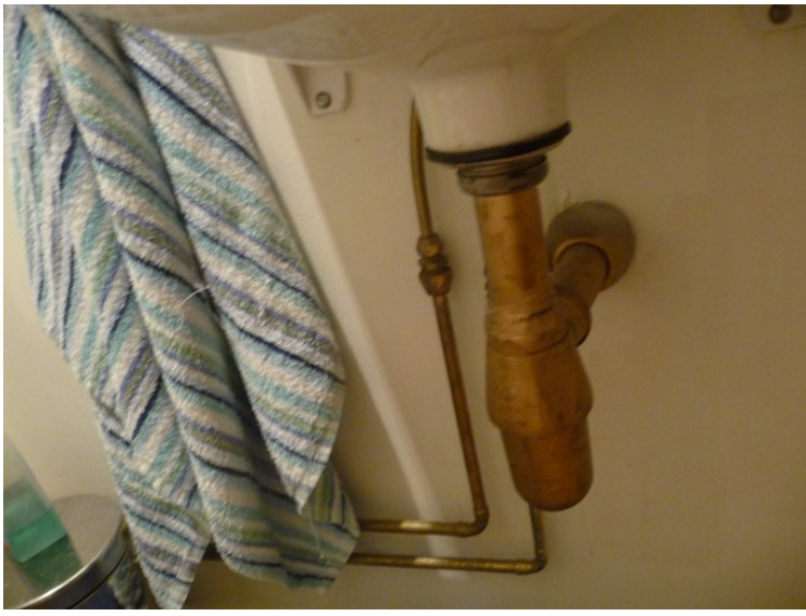
Gold paint on the trap and pipes.
