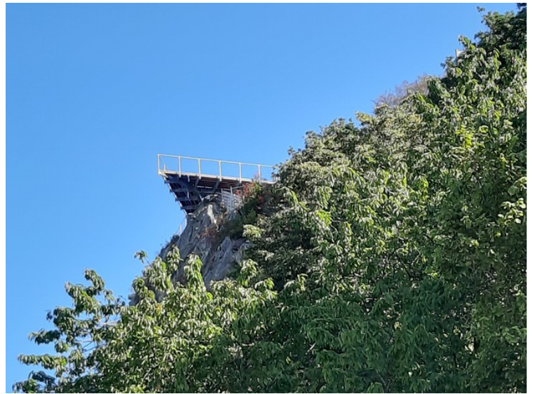
At the top we see a viewing platform that is not finished yet.
