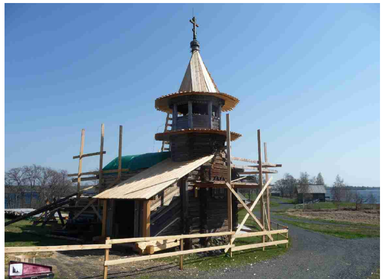
Another church, which was under restoration. We did hear the bells being played in the tower.
