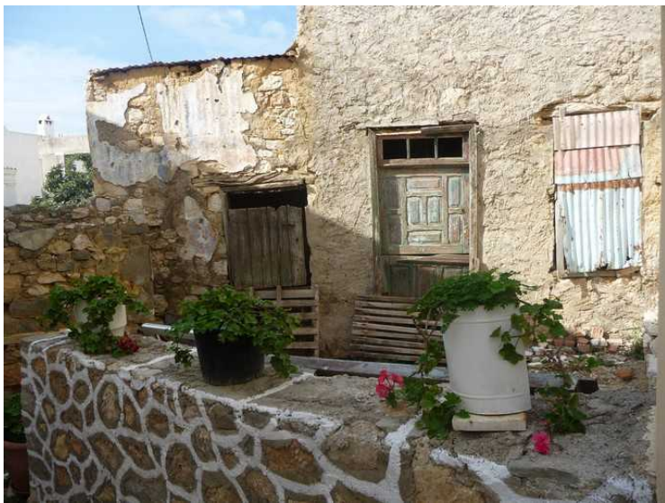
It's nice decorations outside here too, but a little maintenance of plaster and windows, doors and frames is highly needed.
