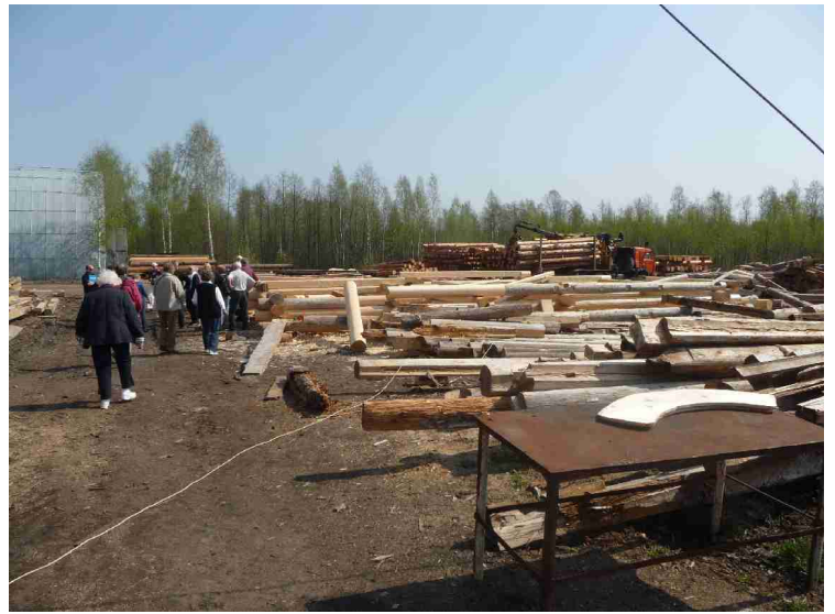
This is the big workshop. They need to be outside when they are restoring houses and churches etc.
