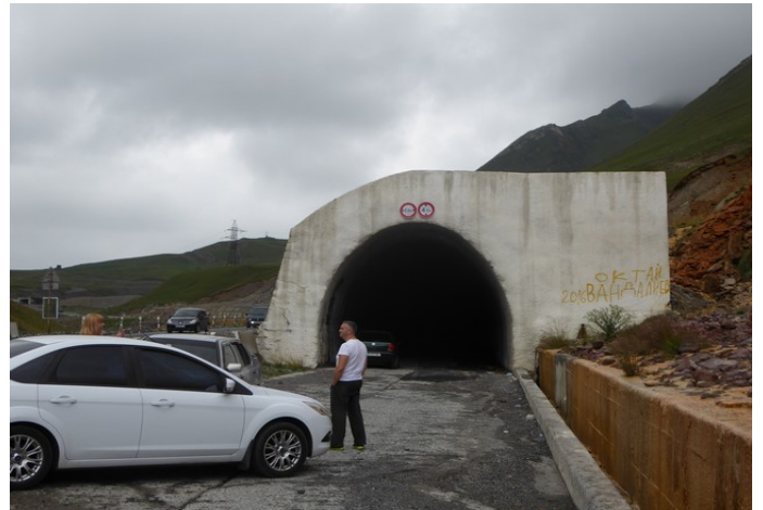
This is a concrete tunnel made along the way, so that it will be possible to drive when snowdrifts are still lying here.
