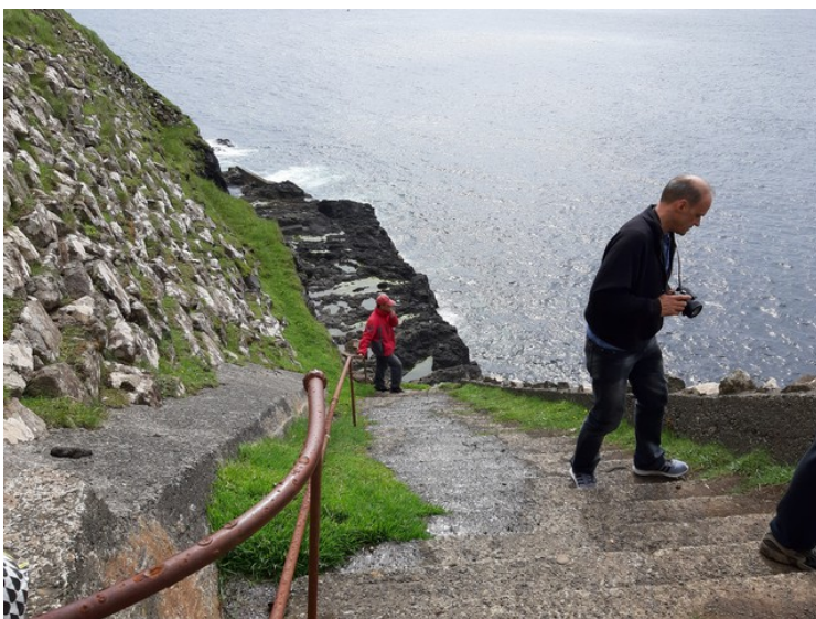
Here the stairs go down. It is stated on the top that it is forbidden to walk in the stairs, but many did not care. The railing was rusty and broken.
