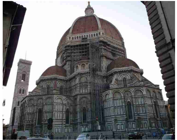
This is the cupola seen from the other side. The dome was at that time the biggest that was made without scaffolding.
