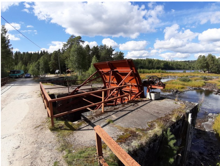
This is the mechanism that operates the dam hatch that can close and open the water.
