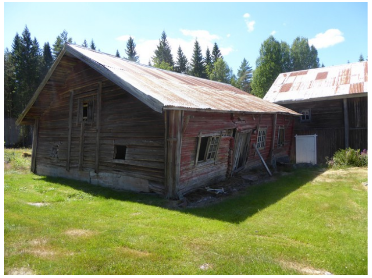
This house needs to be supported so it does not collapse.
