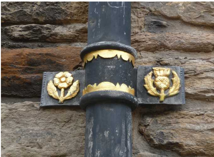
Before going into the Great Hall , we just have to take pictures of the clamps for the drainage pipes from the gutter.
