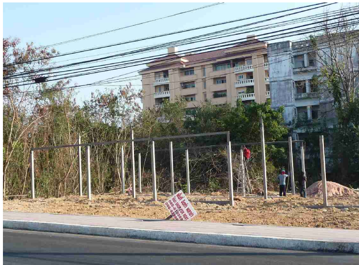
The bush is cleared and pillars are dug directly into the ground in suitable height, such that beams can be mounted at the top.
