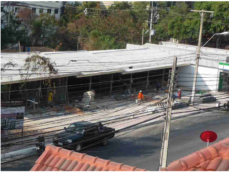
The paving in and out is finished and the brick laying cement has arrived.
