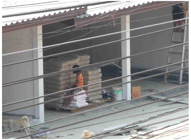
Now the walls are finished, made of concrete bricks, and the painting work has started.
