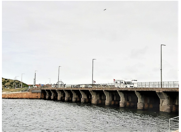
This is the first part of the lock system . It has 14 chambers and is used to regulate the water level in Ringkøbing Fjord.
