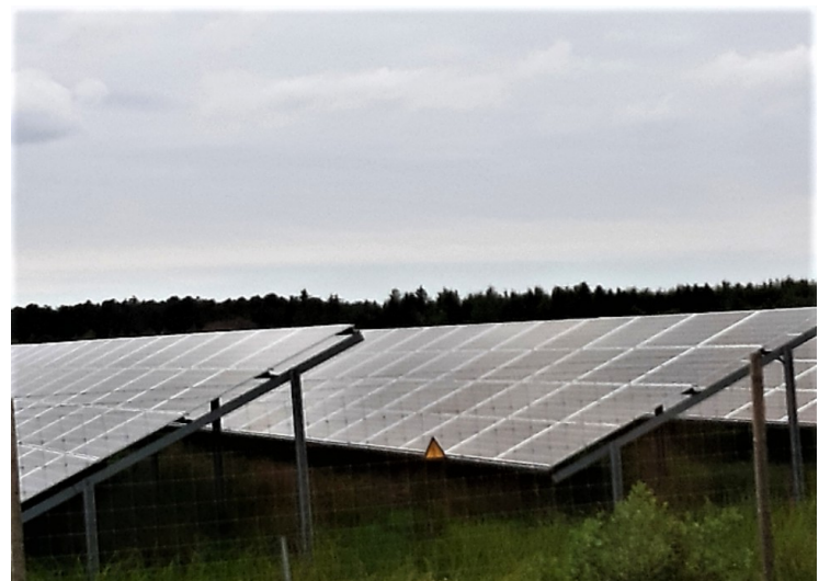
Just south of the city we drove past a large solar cell power plant.
